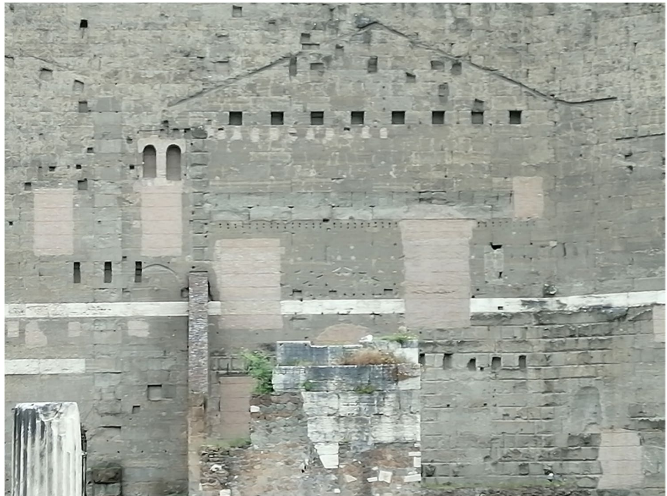
Fig. 6 The perimeter wall that divided the temple of Augustus from the Subura quarter is one of the most imposing peperino works of ancient Rome
