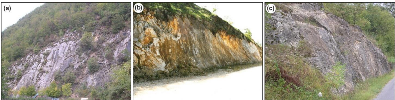
Figure 6. (a) NNW-SSE-oriented fault plane, located immediately above Ascrea village; (b) NNW-SSE-oriented fault plane, near Rocca Sinibalda village; (c) E-W-oriented fault plane, belonging to the Rieti Plain boundary fault system.
