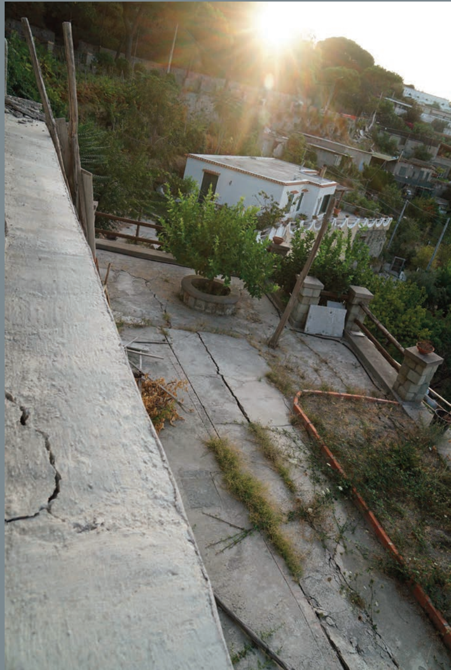
Photo 27 (40.740769° 13.894643°) Coseismic ruptures affecting both concrete basement and ground soil, in a villa along Via Montecito.
