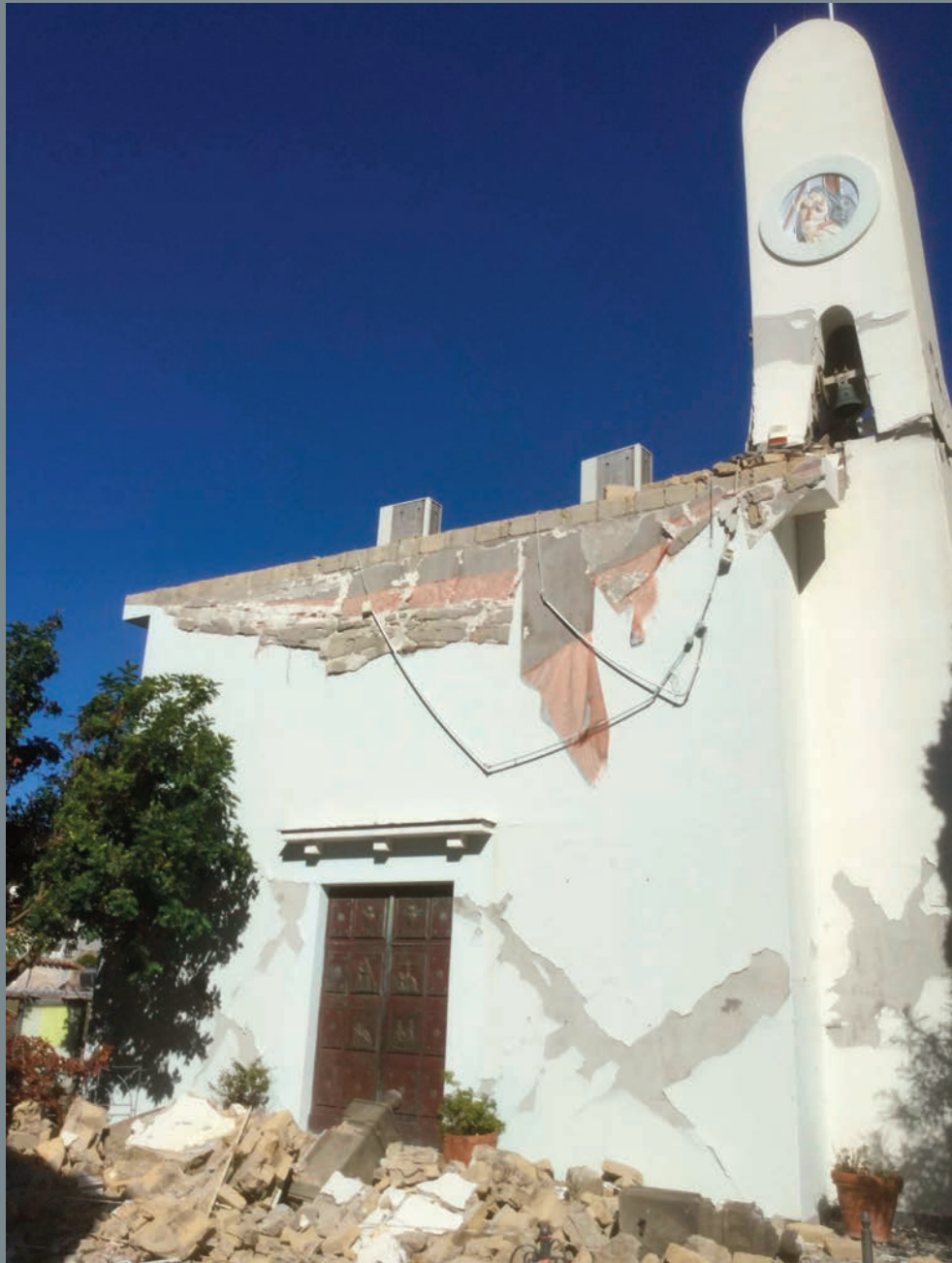
Photo 39 (40.743094° 13.898618°) Severe damages and collapse of the Suffragio church bell tower which caused the death of a woman, along Via D'Aloisio.
