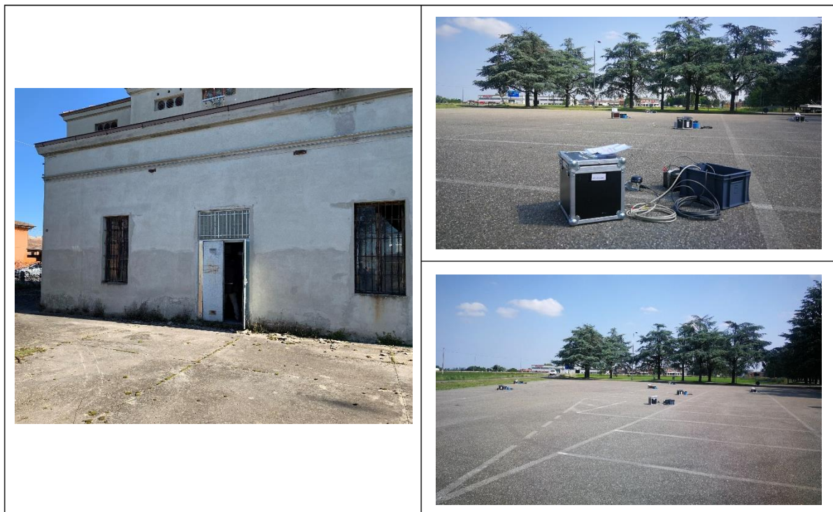
Figure 7: Left: ENEL cabin where the IT.SARM accelerometric station is installed in Sarmato (PC). Upper right: single station ambient noise measurement. Bottom right: 2D passive ambient noise array installed close to the IT.SARM station.
