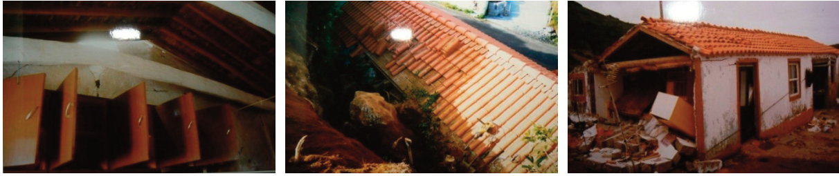
Figure 12. Typical damage to non-structural elements in Azores: a) cabinet doors not latched; b) sliding roof tiles; c) out-of-plan edge walls showing falling cabinets. (Auto de Vistoria post-earthquake survey).
