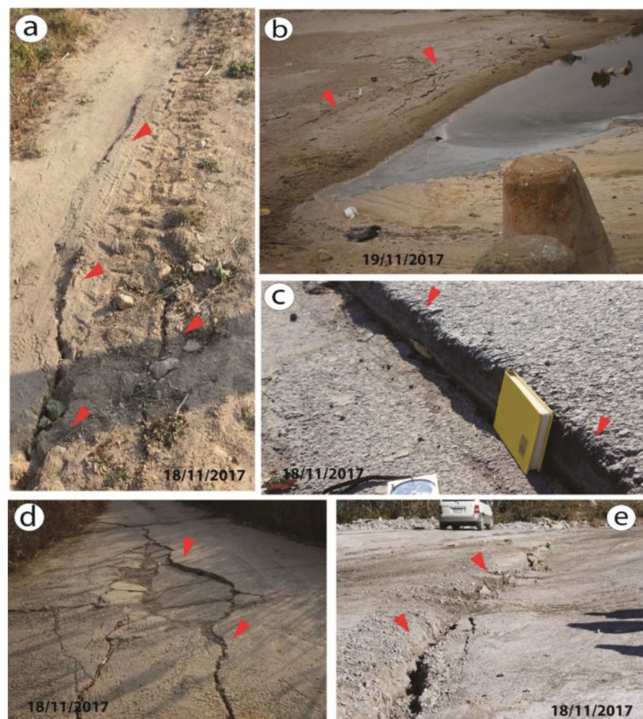
Figure 6. Field photographs showing evidence of lateral spreading observed around the epicentral area of the Pohang earthquake; (a) lateral spreading observed along an embankment of a canal near Yongjeon-ri; (b) evidence of lateral spreading along a sandy beach near Youngil Bay Port; (c) differential settlement due to lateral spreading along a pavement road near Hangdong University; opening of cracks of an embankment near Mangcheon-ri; (d) series of cracks due to slope failure along a concrete road in Mangcheon-ri; and (e) wide openings due to lateral spreading along a reclaimed land site near Hangdong University.
