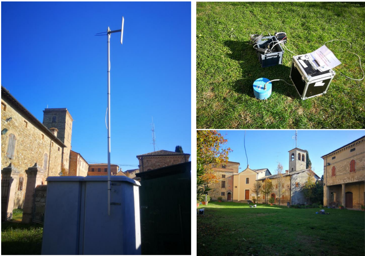
Figure 7: Left: IT.SSU accelerometric station installed on a concrete insulated pillar inside an ENEL transformation cabin (Montegibbio Castle, Sassuolo). Upper right: single station ambient noise measurement performed at IT.SSU station. Bottom right: 2D passive ambient noise array installed close to the SSU station.
