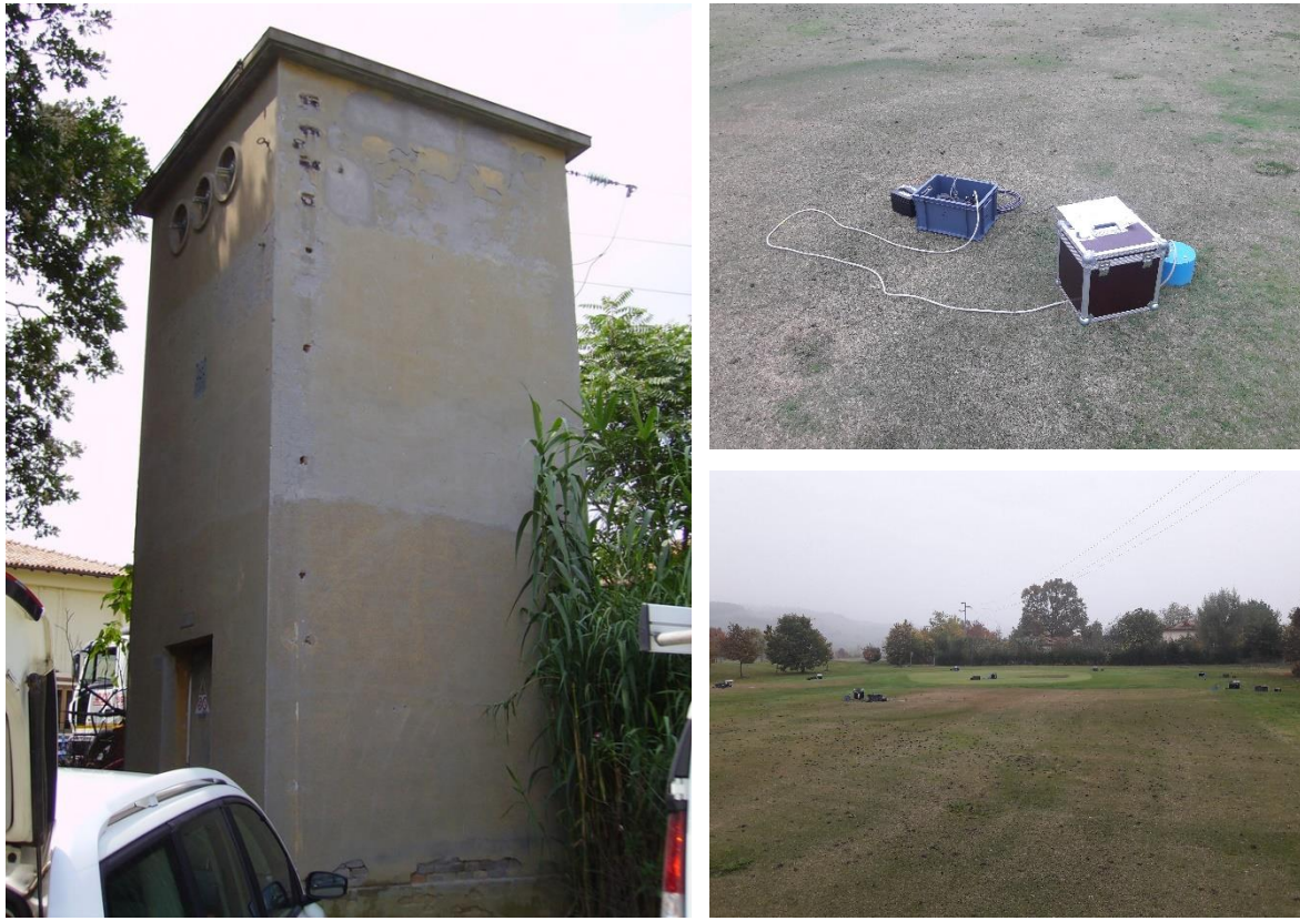
Figure 7: Left: IT.CSP accelerometric station installed on a concrete insulated pillar inside an ENEL transformation cabin (Castel San Pietro Terme, BO). Upper right: single station ambient noise measurement performed at IT.CSP station. Bottom right: 2D passive ambient noise array installed close to the CSP station.
