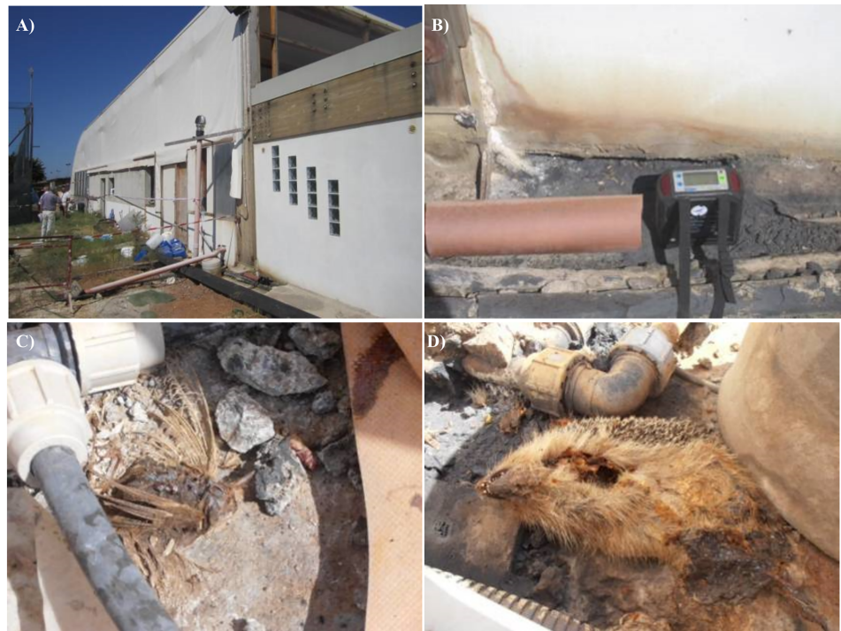
Figure 5. (a) The external southern wall of the technical rooms. (b) Device measuring CO 2 and H 2 S air concentrations. (c) and (d) Evidence of alteration of the metallic parts and dead animals.
