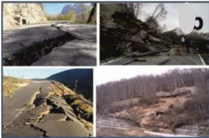
Figure 4 - Landslides on the road, triggered by the EQ.
