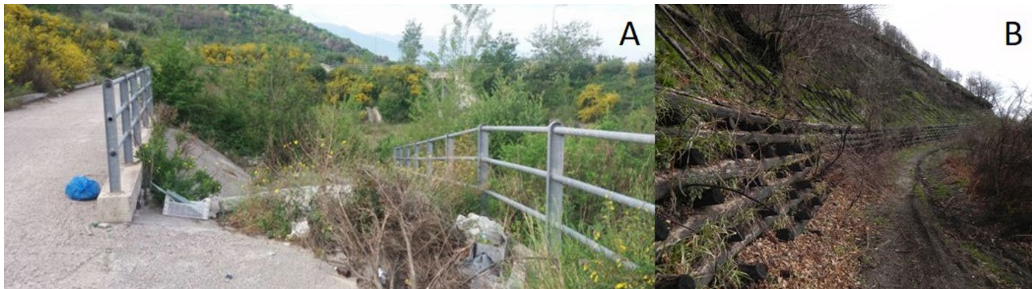
Fig. 19 - (A) Tree trunks and damp at San Vito retention basin ( www.sarnonotizie.it ) and (B) burnt live cribwalls (Sarno).
