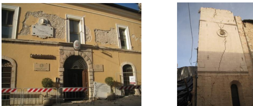
Figure 4 - Damage in Norcia after the October 2016 earthquakes
