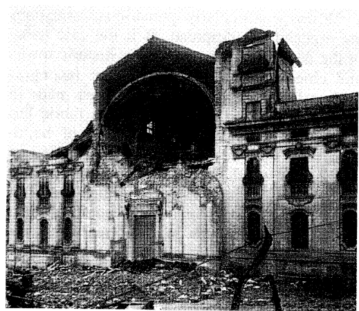
Fig. 4. The front wall of this church was badly built: not well interlocked stones. It was overturned in advance as soon as the horizontal acceleration had concentrated the resultant of the stresses on the edge of the section.
