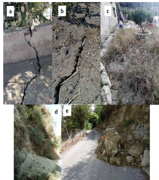
Figure 4: Coseismic surface effects: a) and b) surface rupture in Fango (Lacco Ameno); c) surface rupture in via Montecito (Casamicciola); d) e) landslides in volcanoclastic deposits in Casamicciola.
