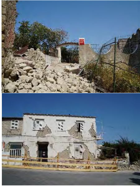
Figure 2: Houses collapsed and heavily damaged by the 21 August 2017 earthquake in the hilly historical centre of Casamicciola Terme (Ischia island). Photos by S. Porfido.
