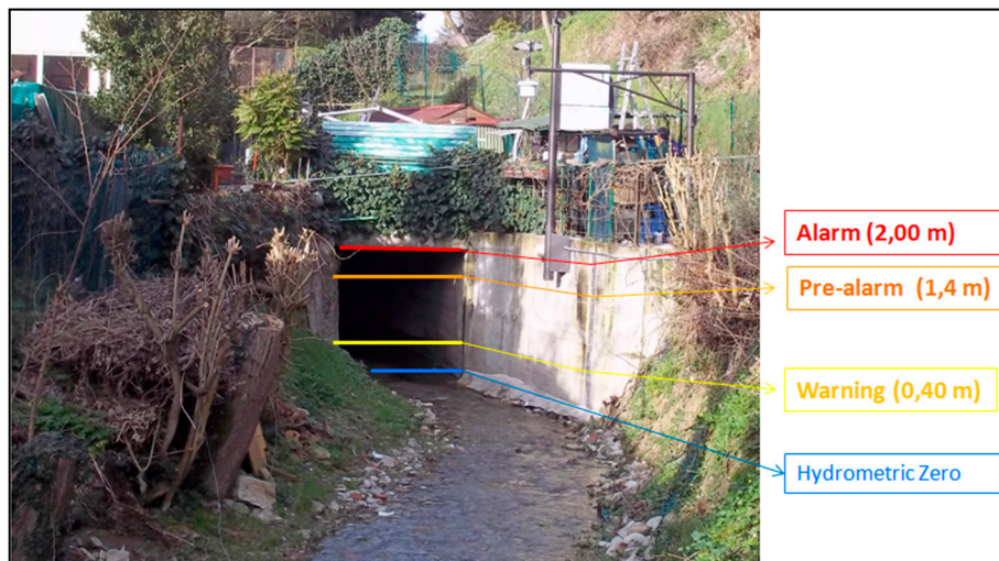
Figure 3. The entry of the culvert of the Ravone creek where the water level gauge is installed and the alarm thresholds are highlighted.
