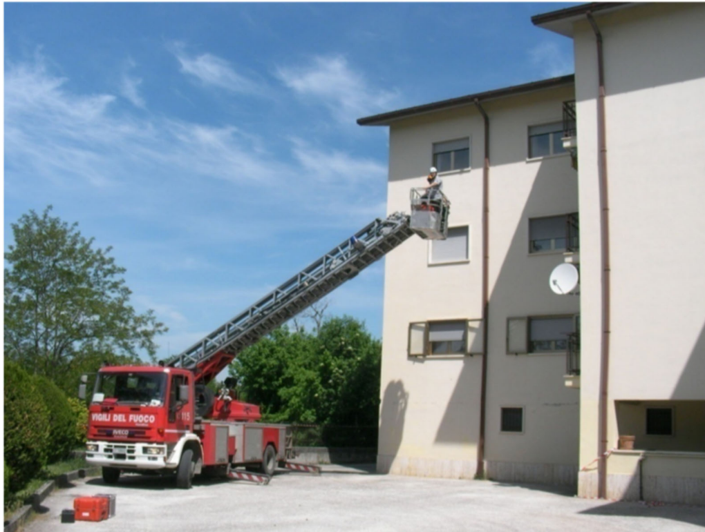
Figure 11: a phase of the installation of the instruments from outside of the buildings using a Fire Brigades truck
