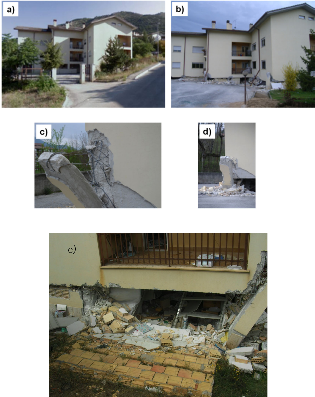
Figure 3: Building A before (a) and after (b, c, d, e) the seismic event
