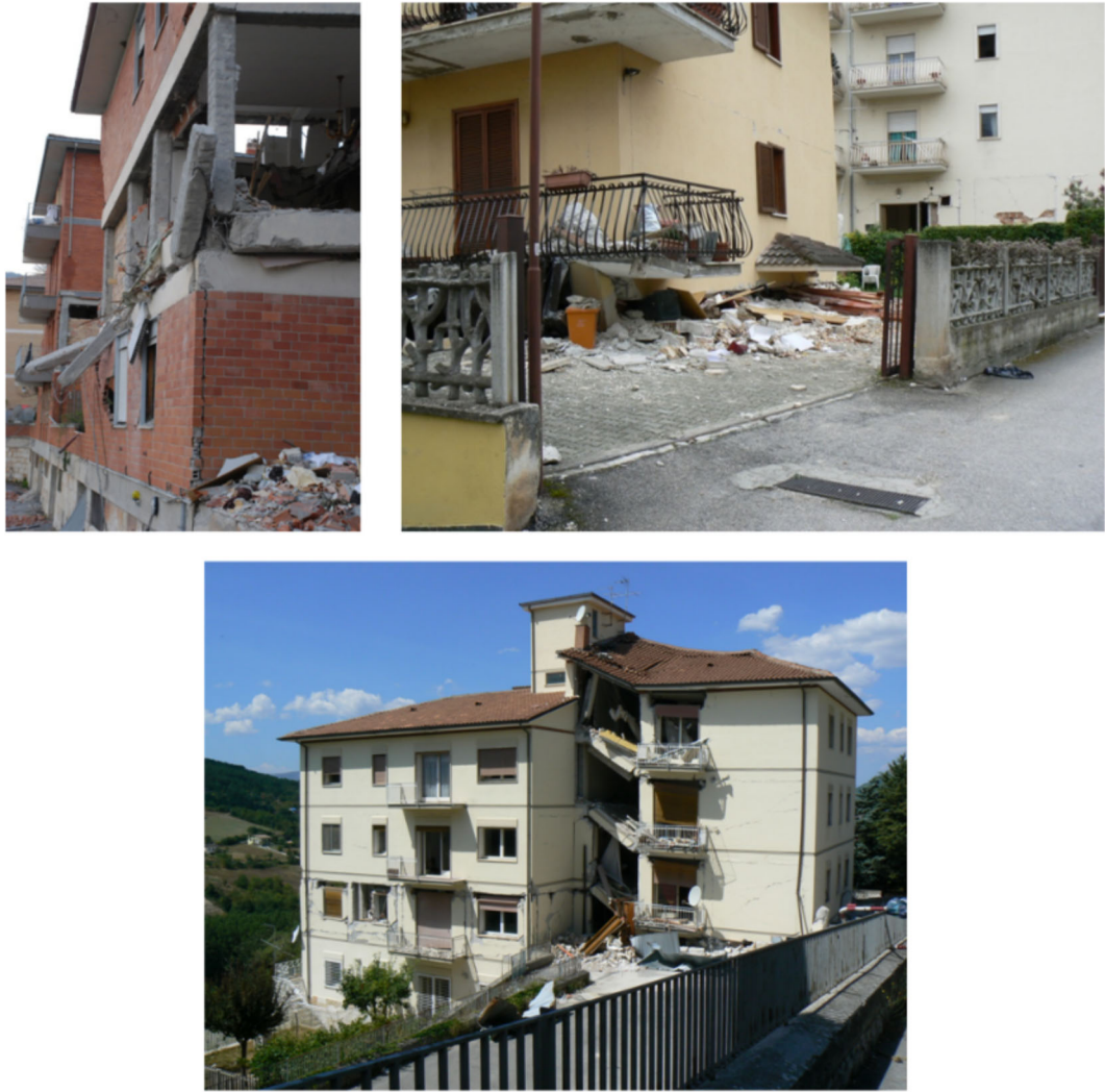
Figure 1: Soft story collapses observed after the 6 April 2009 L'Aquila earthquake
